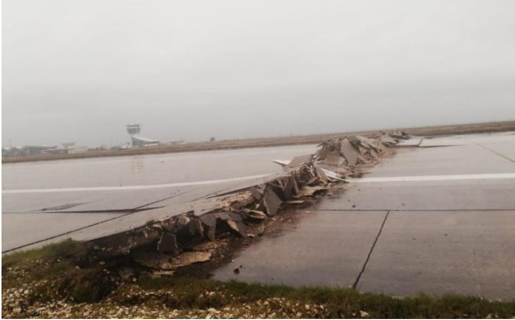
Figure 3. Damage to Hatay Airport
