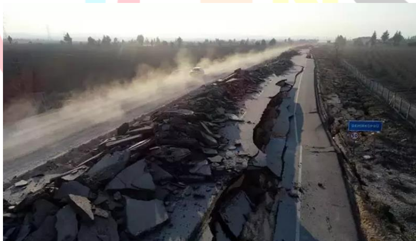
Figure 4. Damage to Antakya Demirköprü Highway (DHA, 2023)
